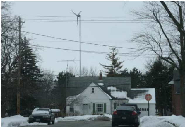
2.4 kW/12 foot rotor diameter/60 foot system height
