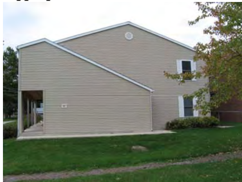
This building façade, while not presenting a blank wall, is not oriented toward the street and is mostly blank. This building is on a corner lot, so a primary entrance is not necessary, but this near blank wall is inappropriate.
