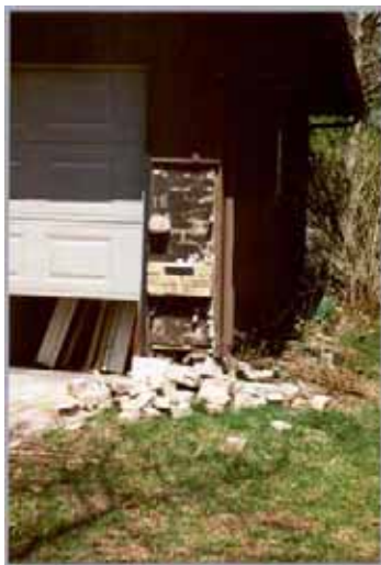
Figure 3.9 Typical Minor Tornado Damage 1996, Urbana
