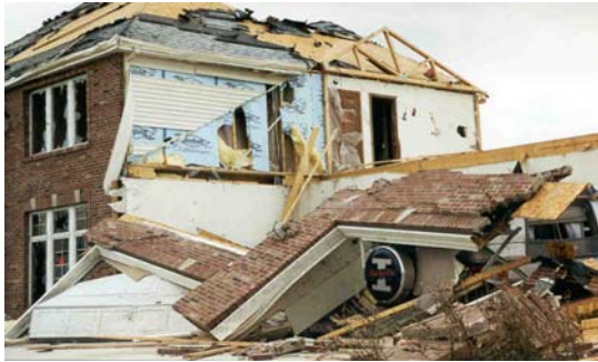
Figure 3.7 Typical Major Tornado Damage, 1996, Urbana
