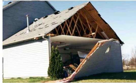
Figure 3.8 Typical Medium Tornado Damage, 1996, Urbana
