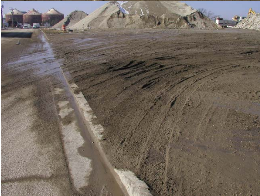
#5: Un-approved curb cut
