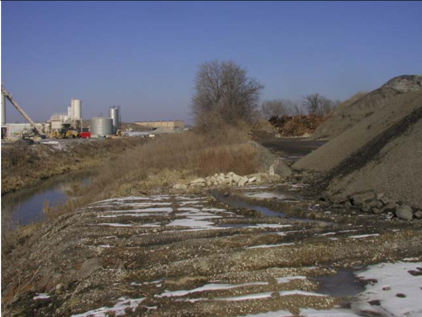
#11: North down Saline Branch bank. Without barriers in front of rocks erosion begins.
