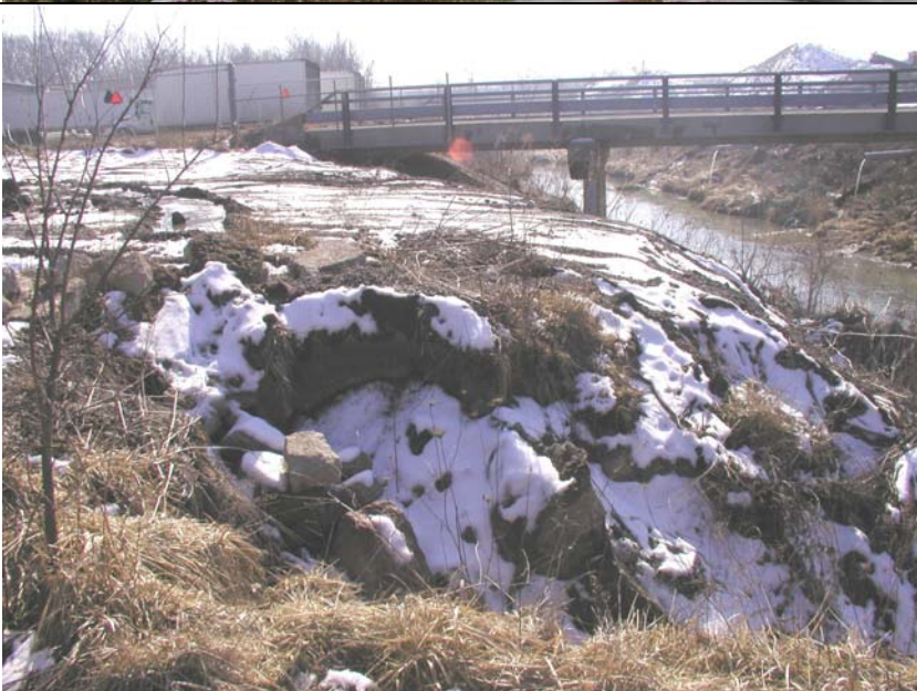
#12: Deep erosion cut of Saline Branch bank without barriers. Rocks at left.
