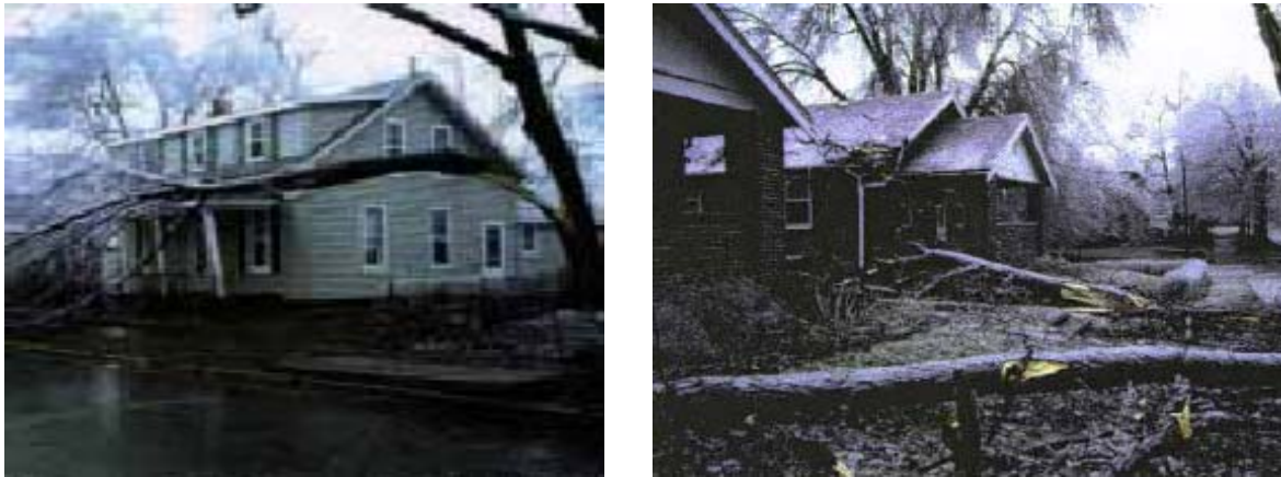
Figure 3.12 Typical Damage from Ice Storm, 1990, Urbana
