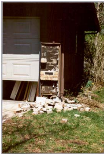
Figure 3.9 Typical Minor Tornado Damage 1996, Urbana
