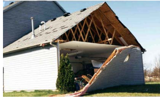
Figure 3.8 Typical Medium Tornado Damage, 1996, Urbana
