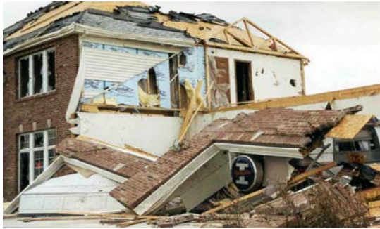
Figure 3.7 Typical Major Tornado Damage, 1996, Urbana
