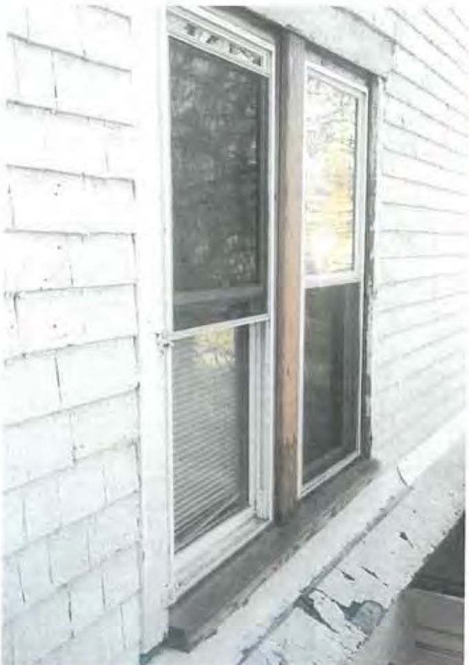
REPLACEMENT WINDOWS & WINDOW TRIM MISSING.
