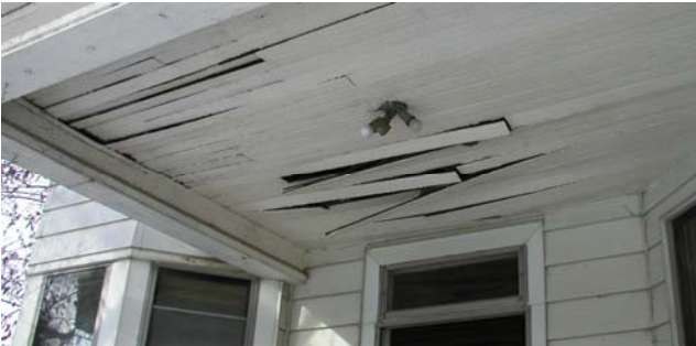
Rotting wood on porch ceiling
