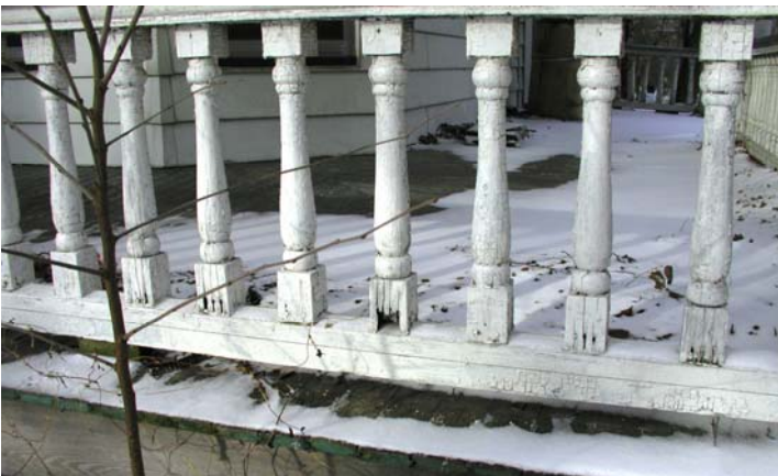
Rotting wood on porch balusters
