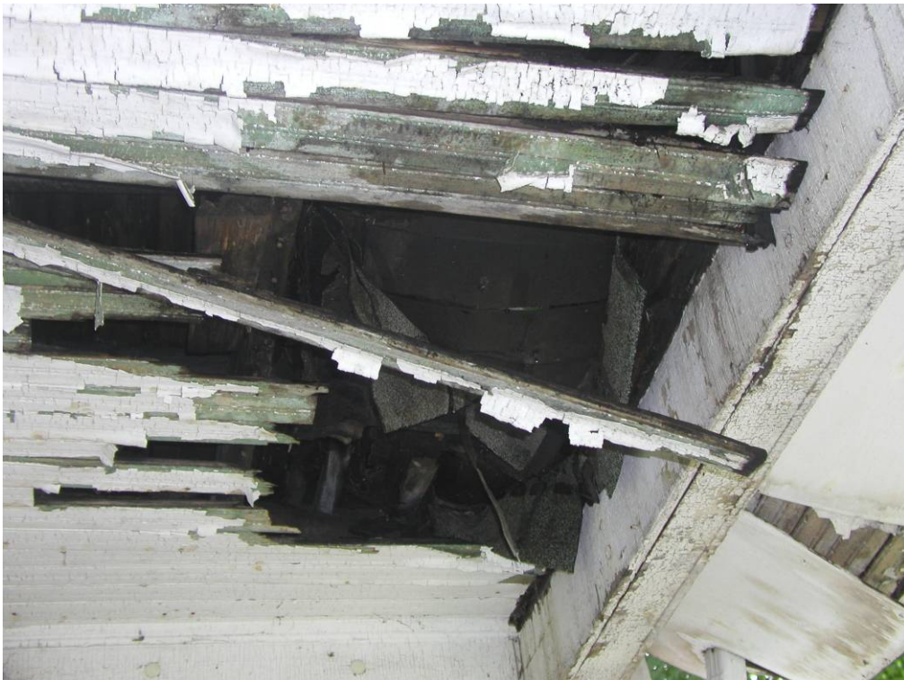
Close-up of damage to porch ceiling
