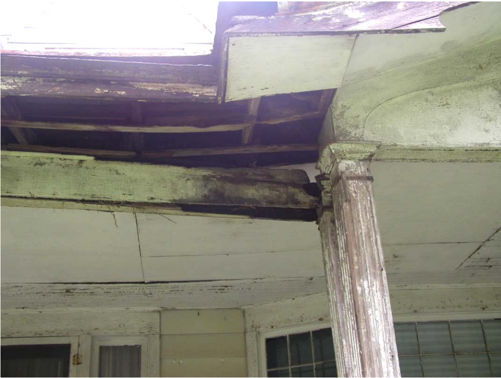
Damage to the structural beams
