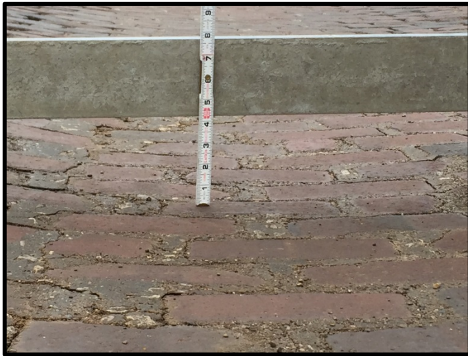
Photo 3: Rutting Depth \pm 4.5''
