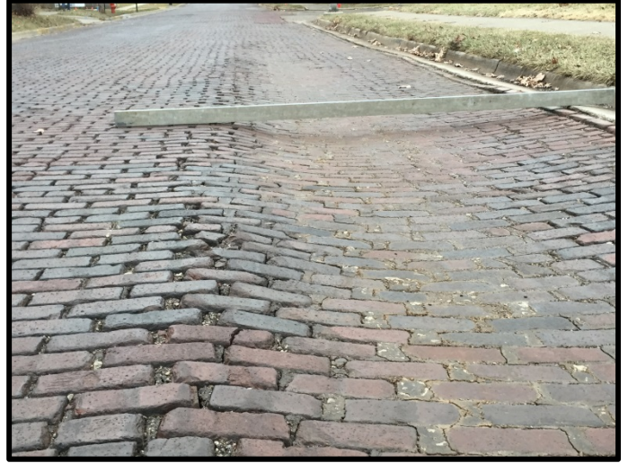
Photo 2: High Severity Rutting
