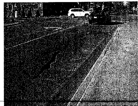
Wright Street Existing Pavement Condition
