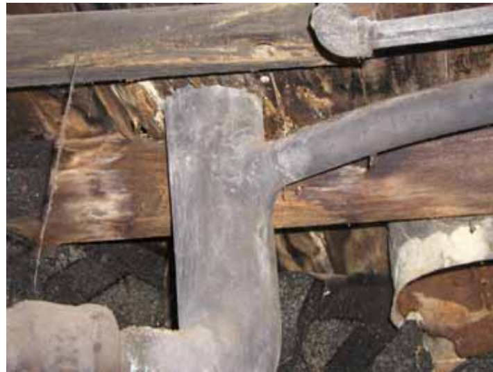
existing plumbing showing long-term moisture damage
