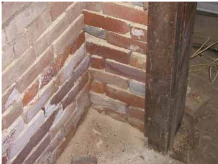
Basement: mortar joints need repointing
