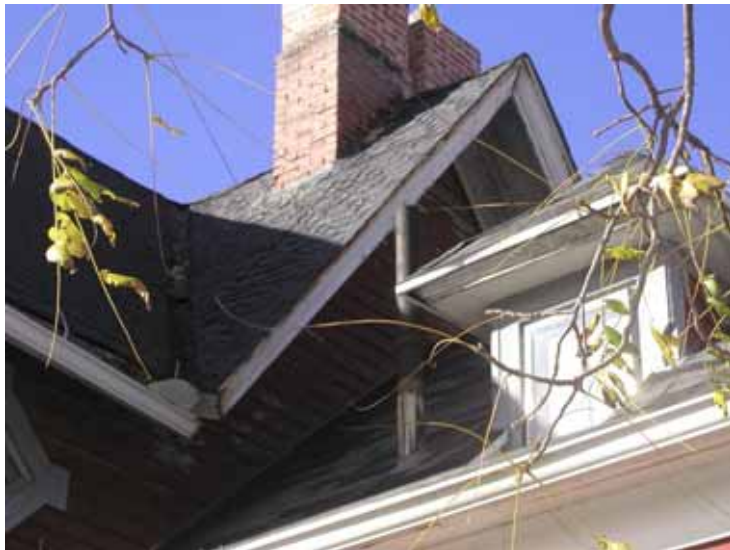
Roof needs replacement
