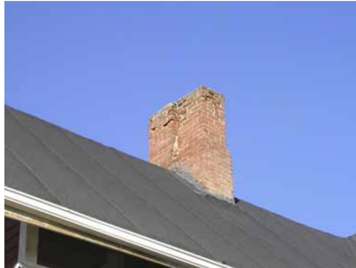
Roll roofing misapplied and minor brick damage to chimney
