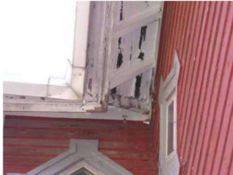
Eaves with failing paint
