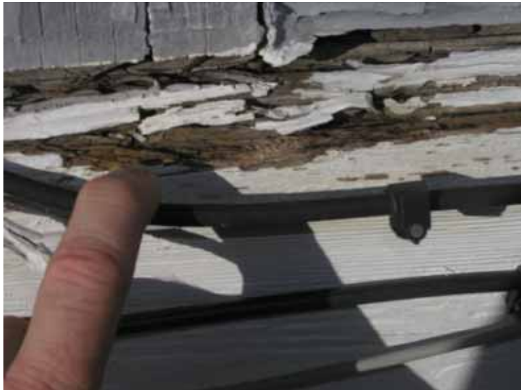
Example of moisture damage around windows
