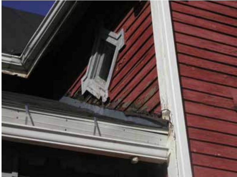
Incorrect roof flashing allows moisture damage
