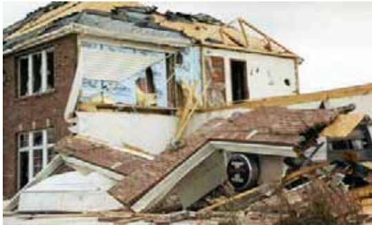
Figure 3.7 Typical Major Tornado Damage, 1996, Urbana
