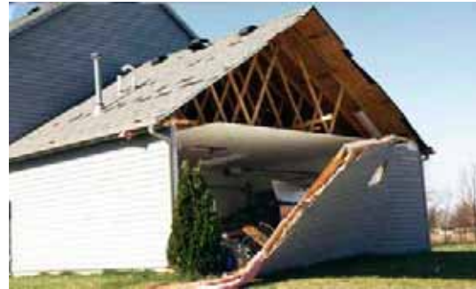
Figure 3.8 Typical Medium Tornado Damage, 1996, Urbana
