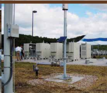
Microturbines at the Sauk County, Wisconsin, landfill.
