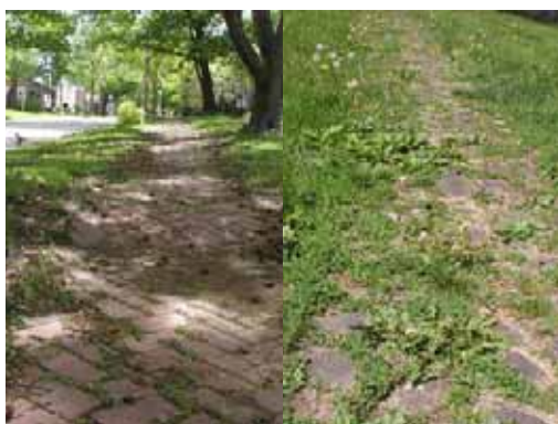
Figure 2. Examples of sidewalks in disrepair.
