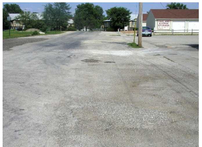
Uneven and poor pavement, potholes on Oakland
