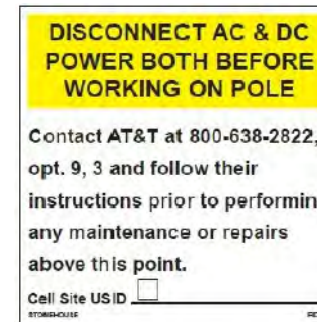
EXAMPLE CRAN POLE POWER DISCONNECT SIGN
