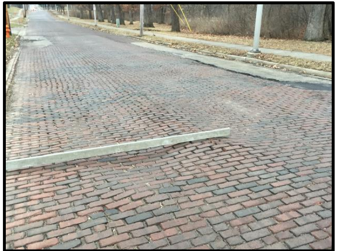
Photo 4: High Severity Rutting & Low Areas Patched With Asphalt
