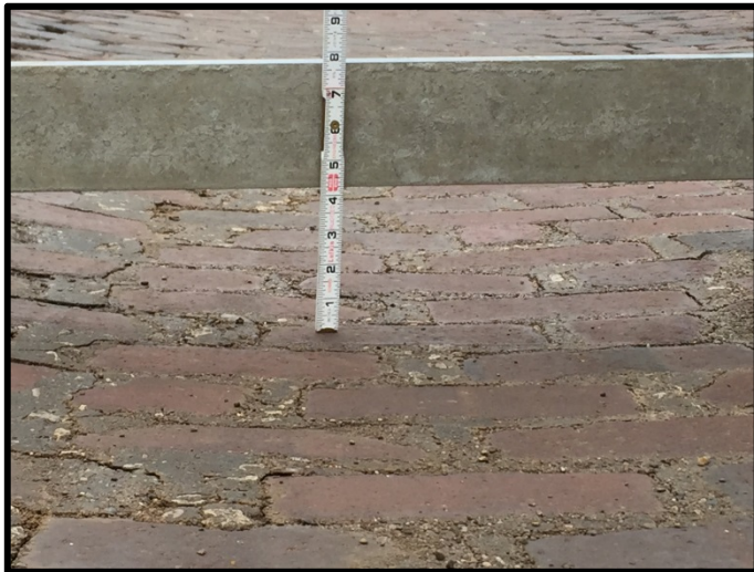
Photo 3: Rutting Depth \pm 4.5''
