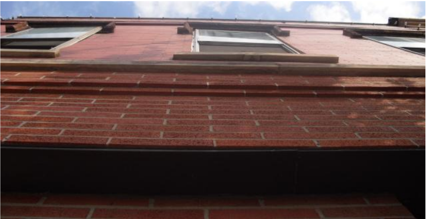
Photograph #2: The second story wall is bowed.
