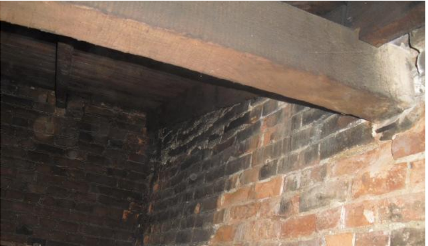
Photograph #4: Poor condition of Interior Brick Wythe, west end of South Wall
