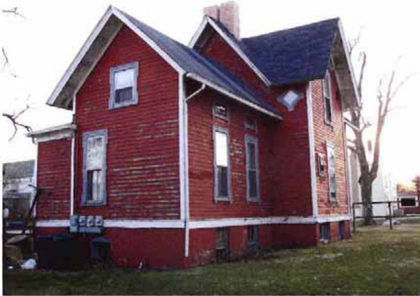
View of north and east elevations. The view is towards the southwest.
