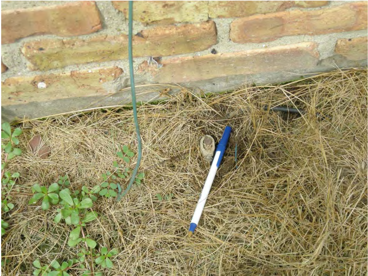
807 Mattis; Multiple Dwelling Unit; Grounded, but rod too thin and no bond to building ground system; not OK
