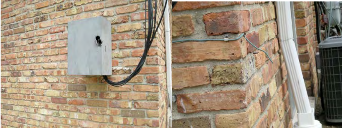
809 Mattis; Multiple Dwelling Unit; No ground connection; not OK.
