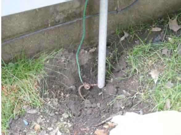
507 W. Green; Old box hanging; ground OK.
