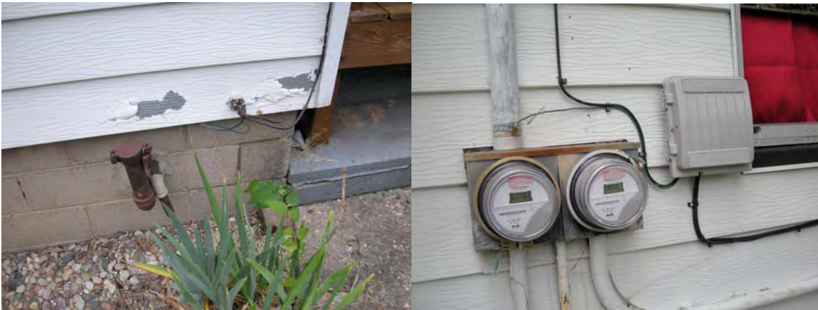
506 W. Green; two cable television drops; the one with the box has a ground clamp for which the paint was not scraped off very well.
