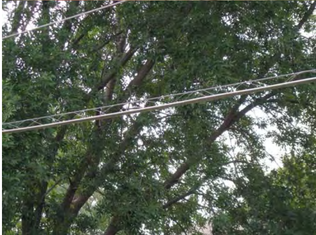
907 Mattis; Multiple Dwelling Unit; No ground connection; broken lashing wire on cable behind building; not OK.
