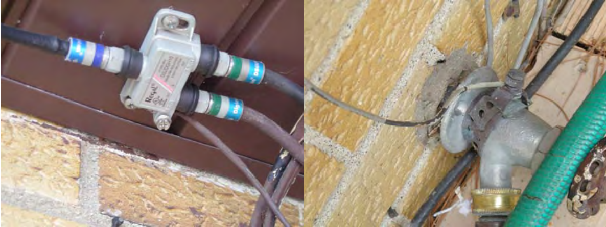
1010 Broadmoor; Loose pipe strap on hose faucet; not OK.
