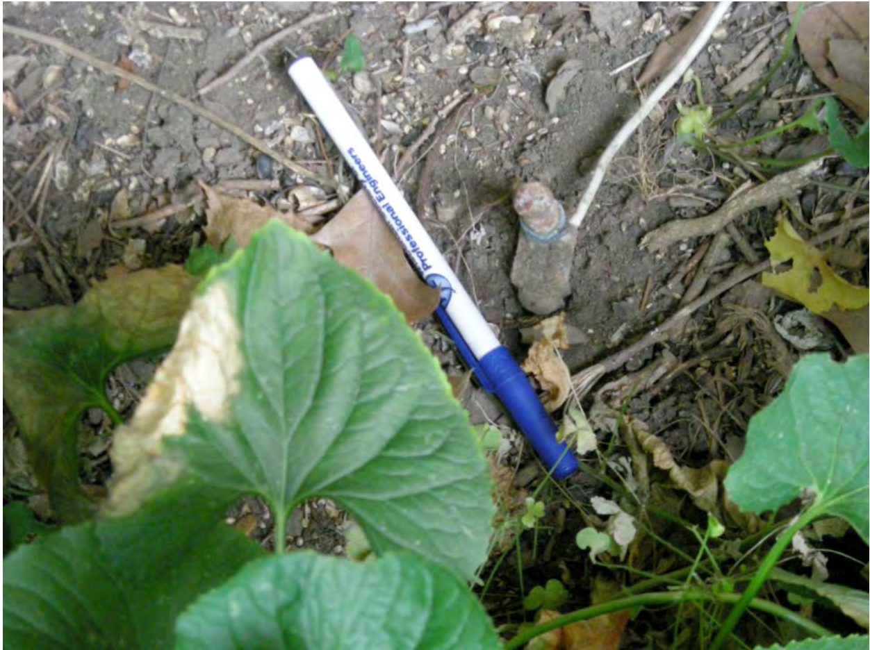
1206 Broadmoor; Ground rod too thin and not bonded to building system ground; not OK.
