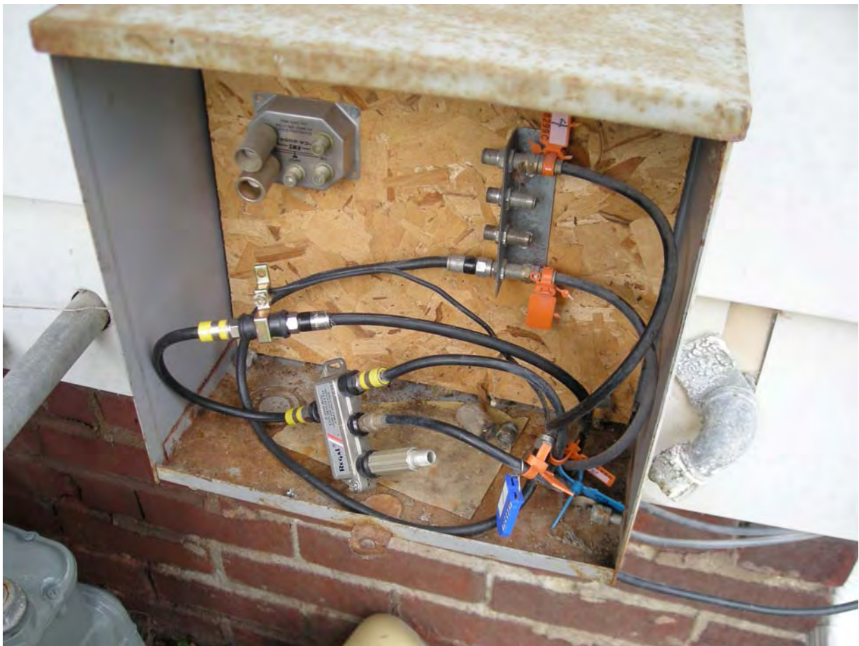
604 S Race; Multiple Dwelling Unit; ground OK; box missing cover; ground wire enters building; unable to enter building to check.
