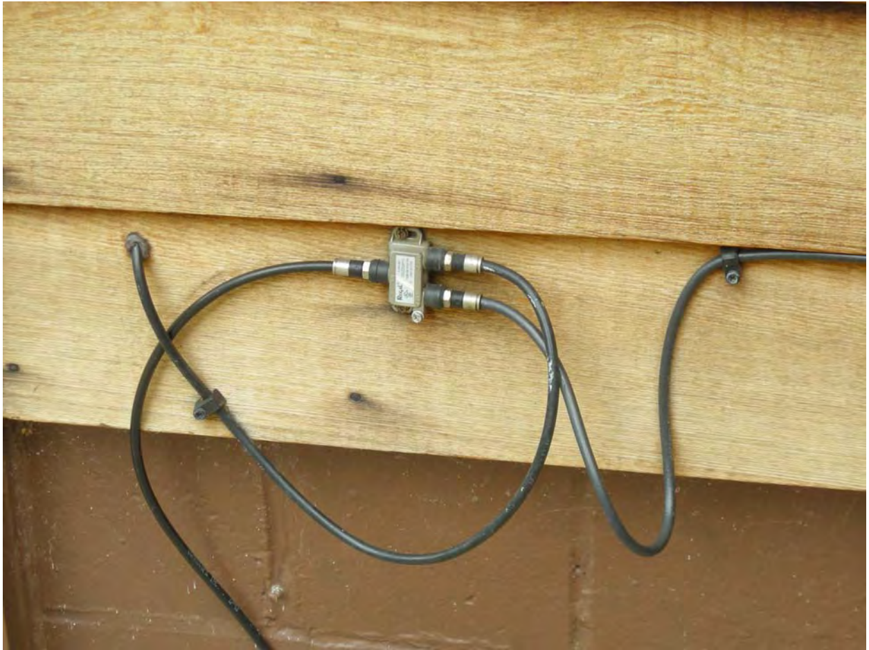
1802 Crescent; No ground found; not OK.
