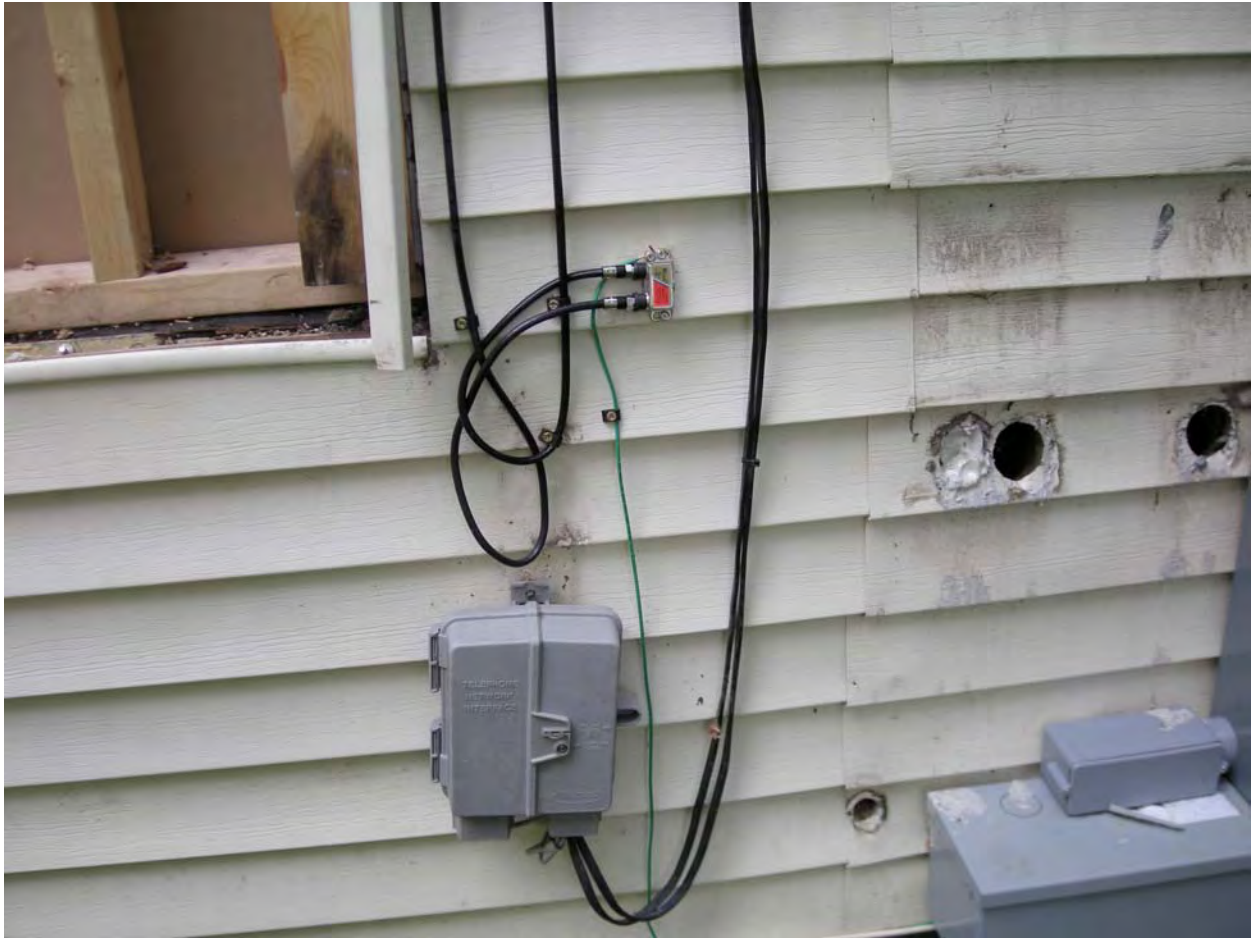
606 S Race; ground wire enters building; no response, unable to enter to check.
