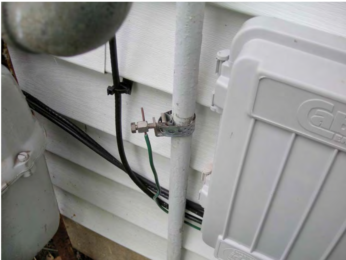
1603 Wiley; not very good job of scraping paint off conduit; otherwise OK.
