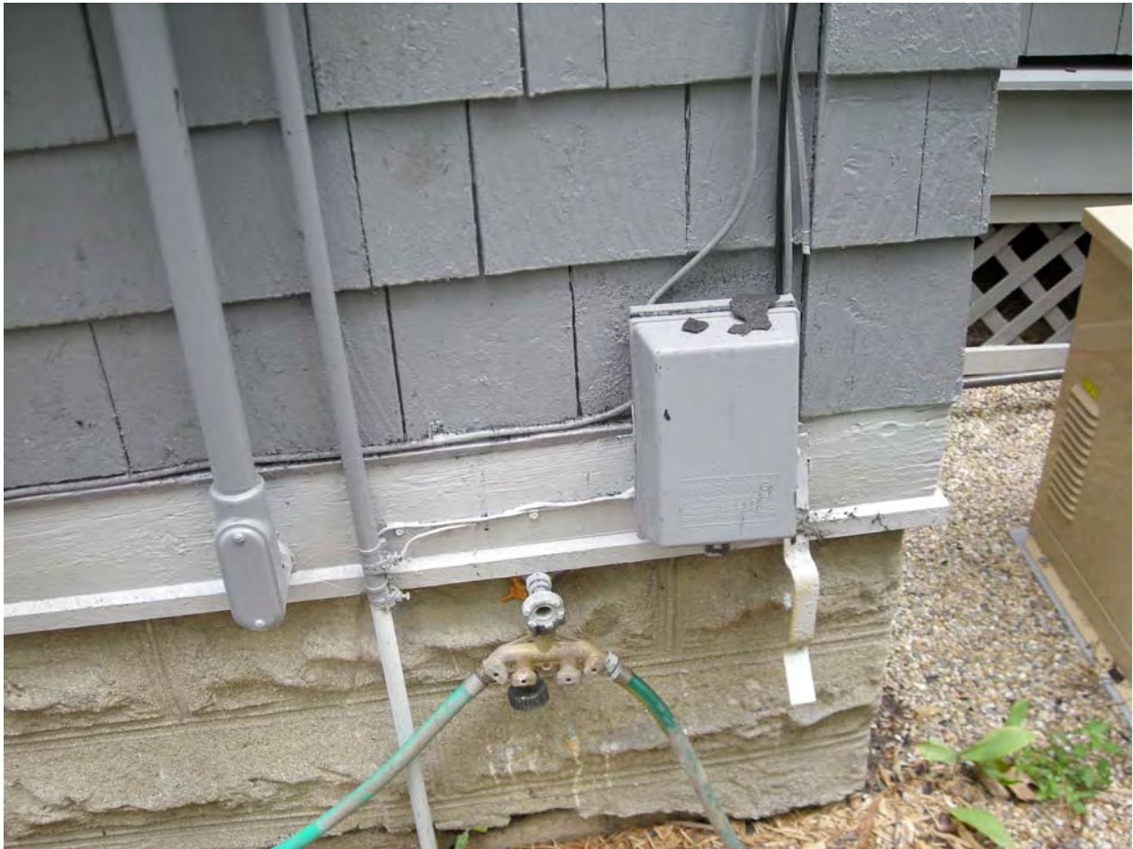
311 W Washington; remodeling taking place; no cable television ground or bond found.
