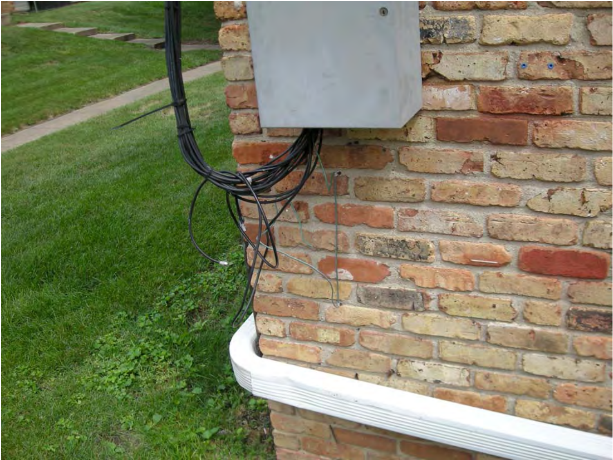
903 Mattis; Multiple Dwelling Unit; No ground connection; not OK
