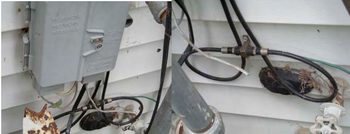
1004 Delaware; grounded to the ground rod used for the building electric ground; ground is OK.
