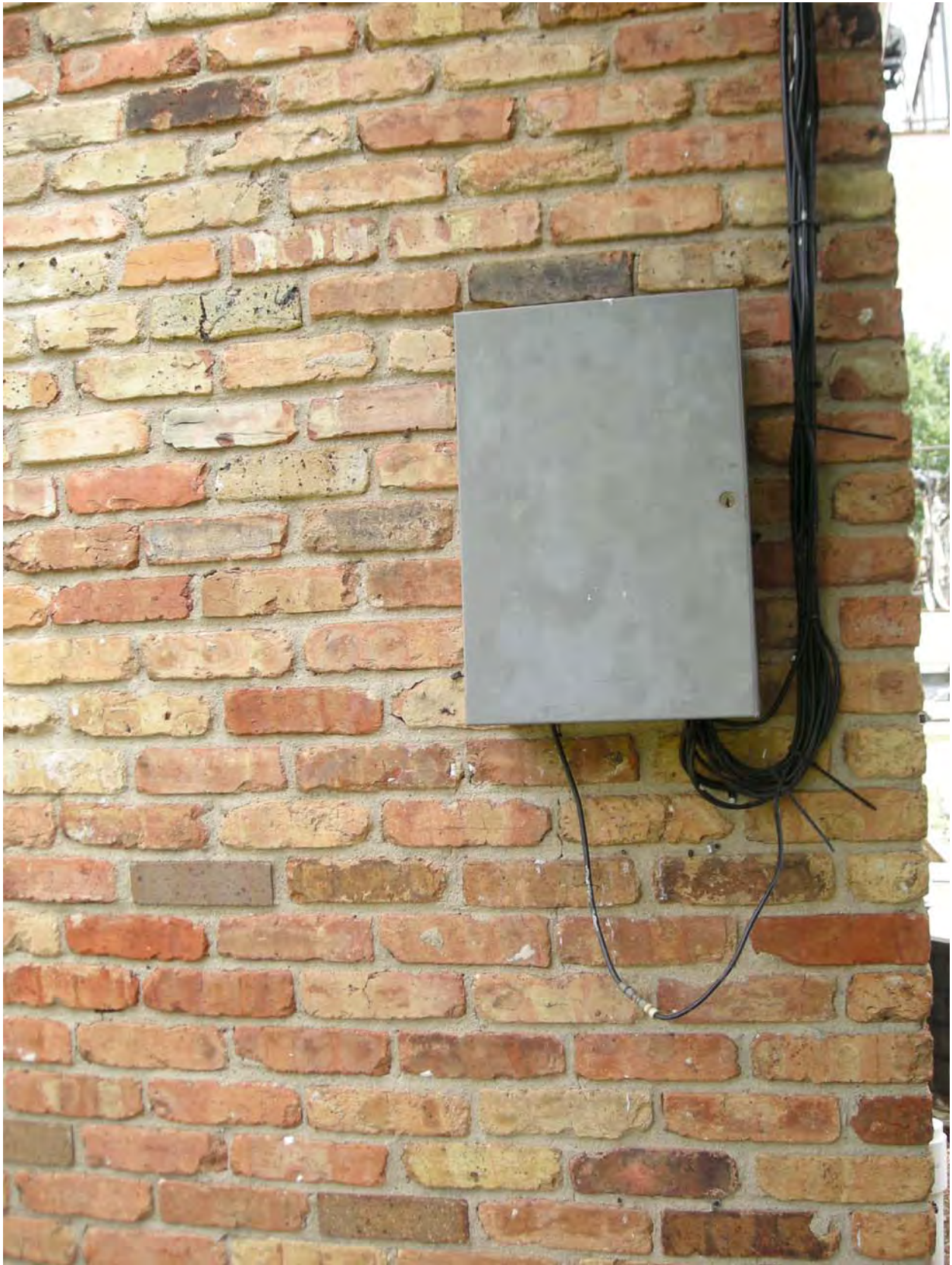
911 Mattis; Multiple Dwelling Unit; No ground connection; not OK.
