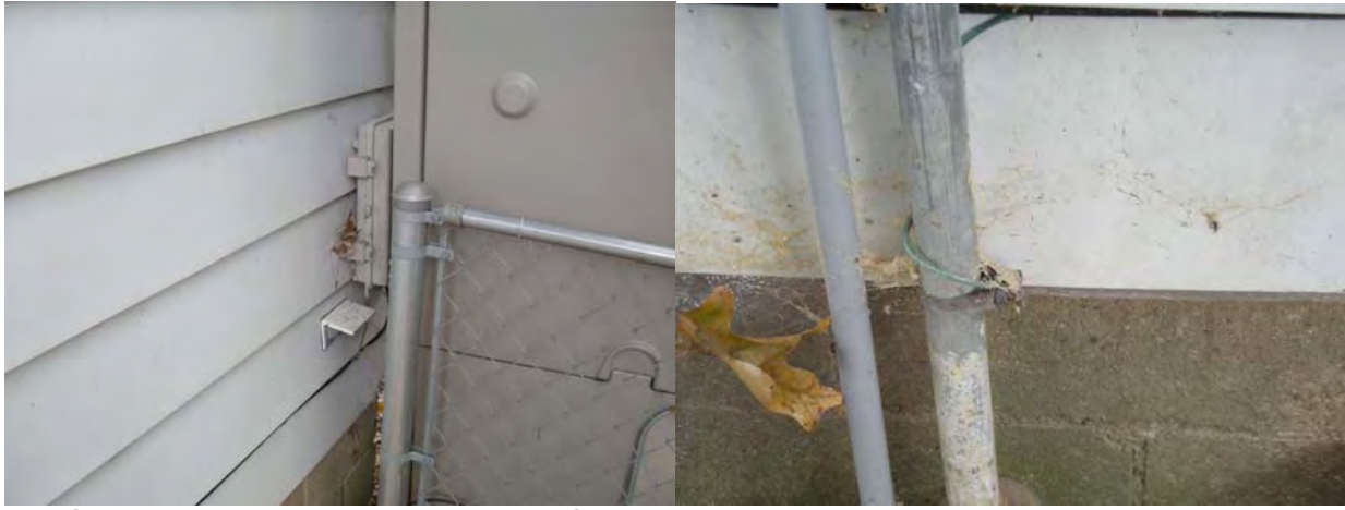
806 S Weber; Bond to power entrance; OK.
