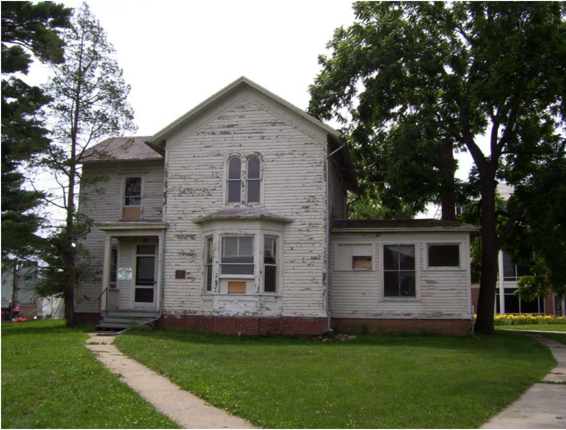
View of Mumford House looking south. (Buell Hall is to the far right.)
