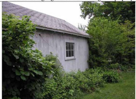
#10 East wall of garage on lot line from neighbors yard.
