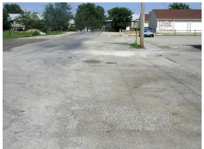
Uneven and poor pavement, potholes on Oakland
